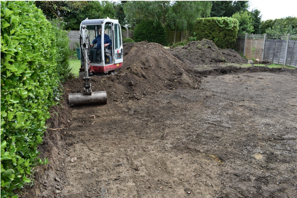
View 1. View of site of the area for foundations of the proposed house
