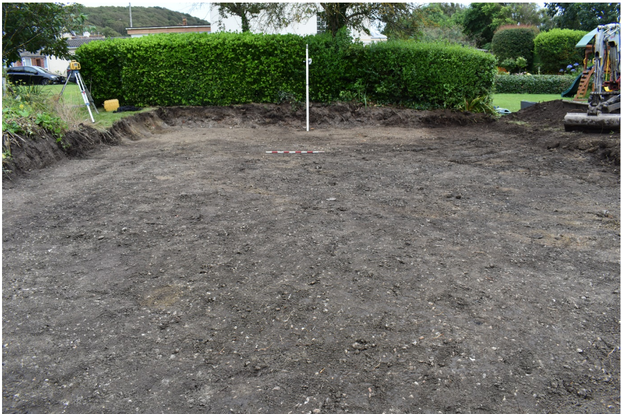
Plate 1. View of the site after Phase 1, clearance of the topsoil (looking ENE)
